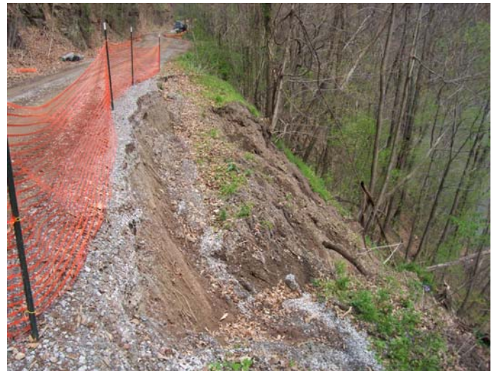
Slope Failure—7 Total Slide Areas
