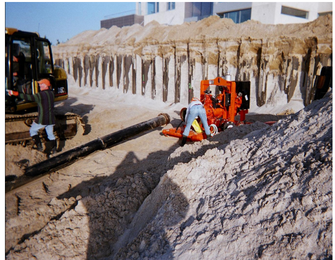
Steel Sheet Bulkhead left exposed from the storm
